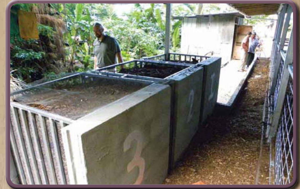
Closing the cycle. The integrated composting system is an important design element of the dry litter technology.
